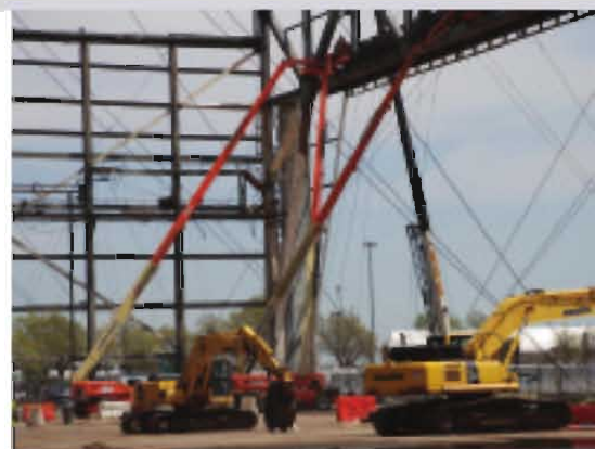
The cover and roofing of the JFK East Hanger Extension had already been removed. The frame consisted of two steel frame walls connected by two steel trusses
