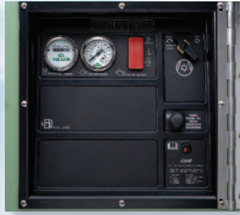
Curbside Instrument Panel with (SSAM) Shutdown System & Annunciation Module.
